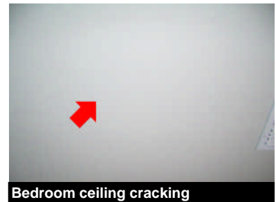
Bedroom ceiling cracking
